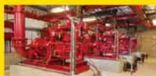
Static Fire Pump
