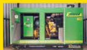
Generator Power System
